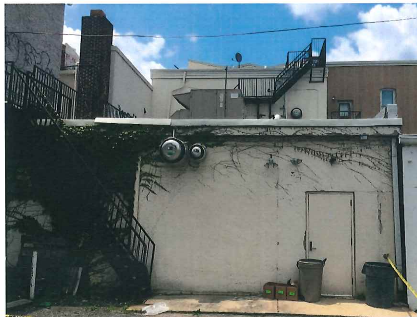
Figure 3: Locating a building's mechanical equipment on the rooftop can shield it from flood damage. In this example, the equipment is located toward the rear of the building, screening it outside of view from the front of the building and commercial corridor.
