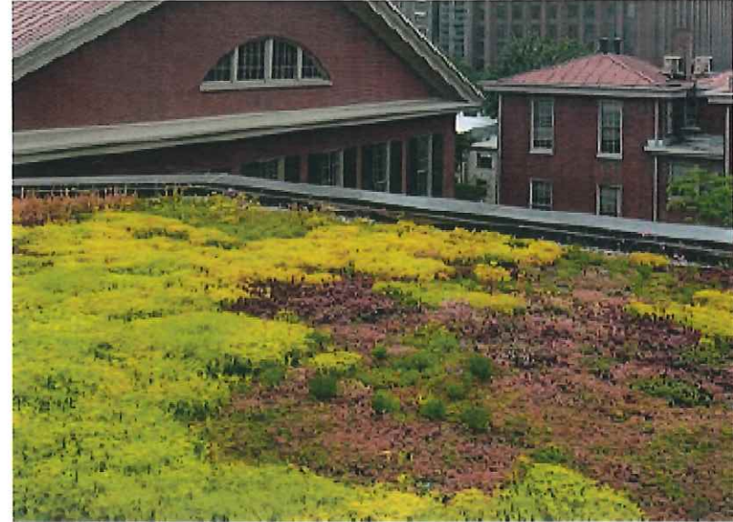
Figure 4: Example of a vegetated or "green" roof
